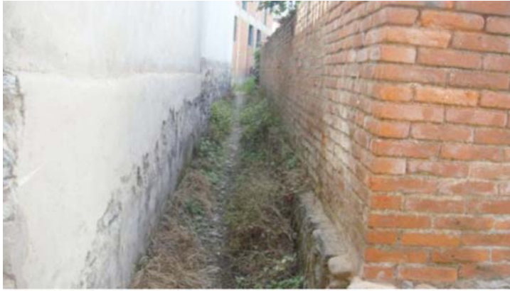
Some parts of the stream inside the village have already dried out.
