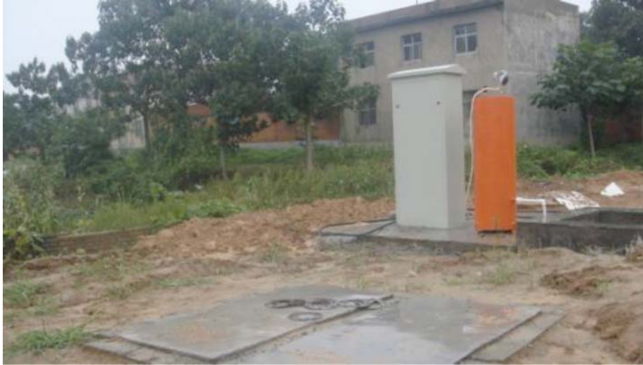
In the middle of 2011, a new well was installed by the local government. We were told by local residents that because of the decline of the water level, the new well has to pump water from a depth of 280 metres under the ground.
